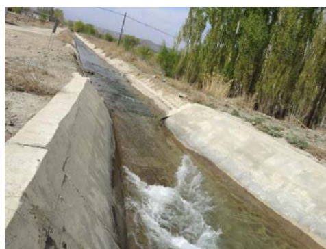
区块北侧头工干渠
